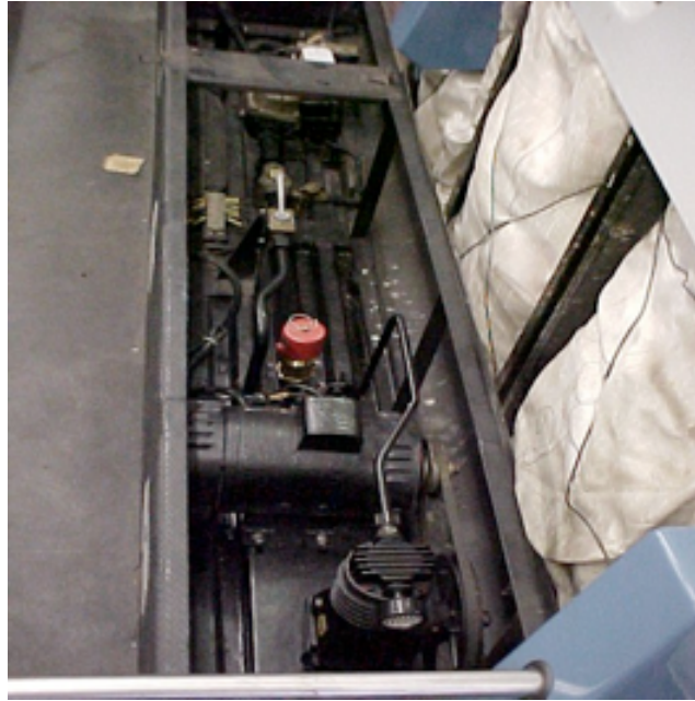
Figura 3-20. Compressor Auxiliar (CBTU/METROREC, 2009).
